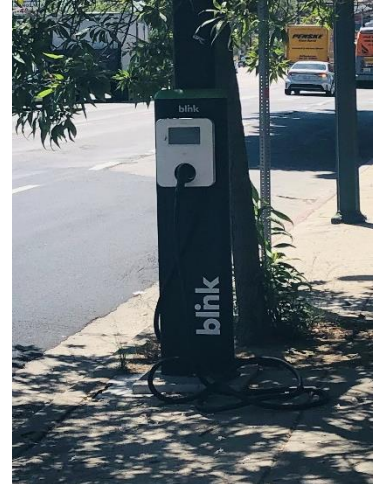
Figure 3. Sample Curbside EVCS
